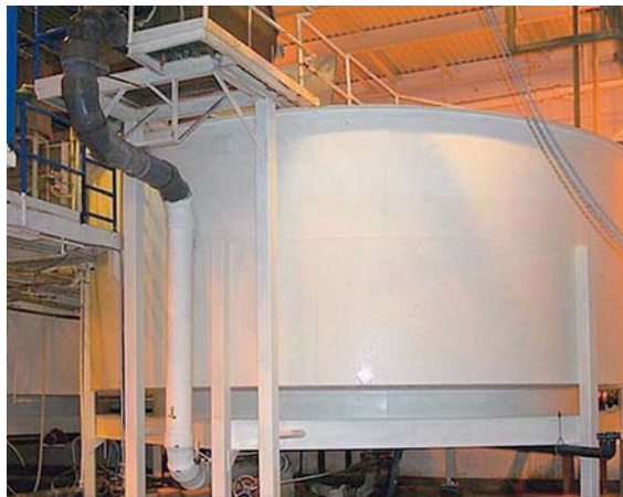
Fig. 2.24 Large, insulated acidulation and extraction tank for gelatine.
